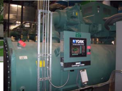
New Chilled Water Plant
