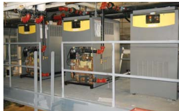
↑ New Condensing Hot Water Boilers
