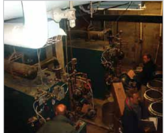
Top and center, the Authority's Lenox Street steam plant and steam controls. Above, the boiler room at Holgate.
